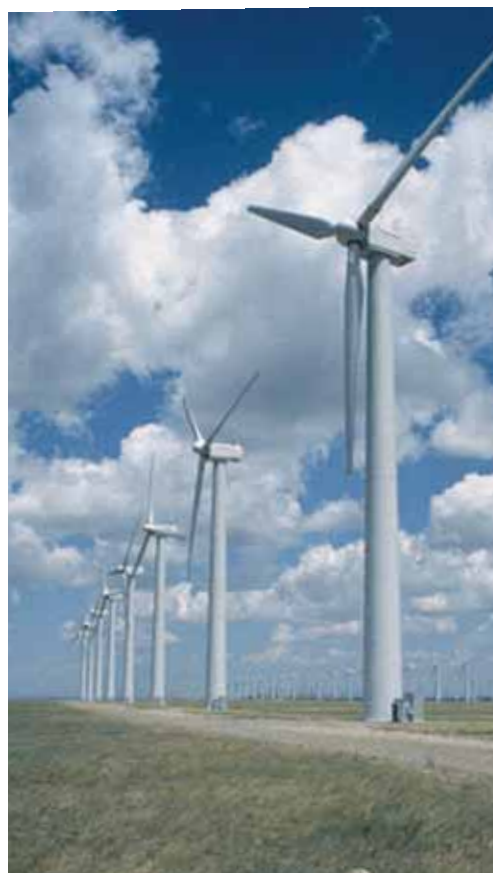
Photo: Eugene Water and Electric Board
